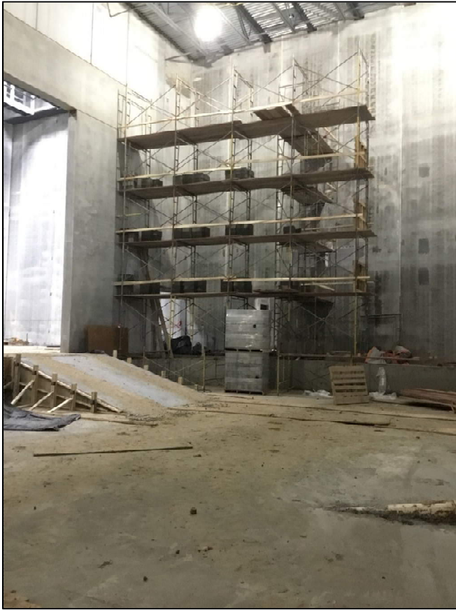
The masons are preparing to build the PAC cheek walls. After these walls are built, the side circulation concrete can be poured.
