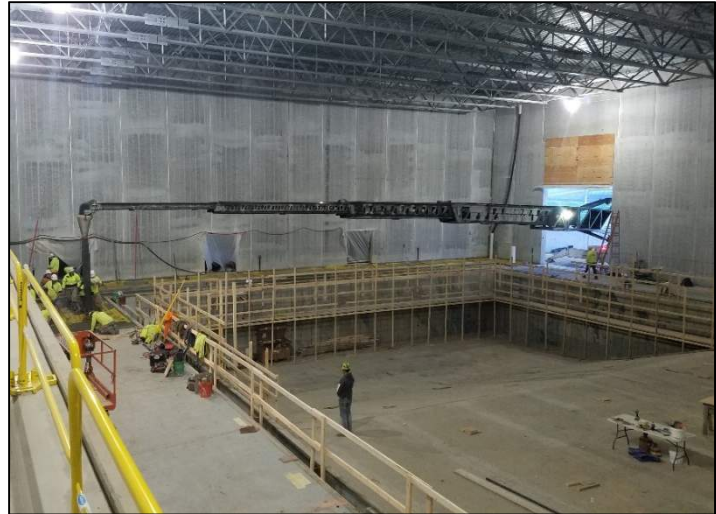
Due to limited access in the Pool, a conveyor was used to pour the final segment of concrete. This conveyor spanned just over 100 feet!
