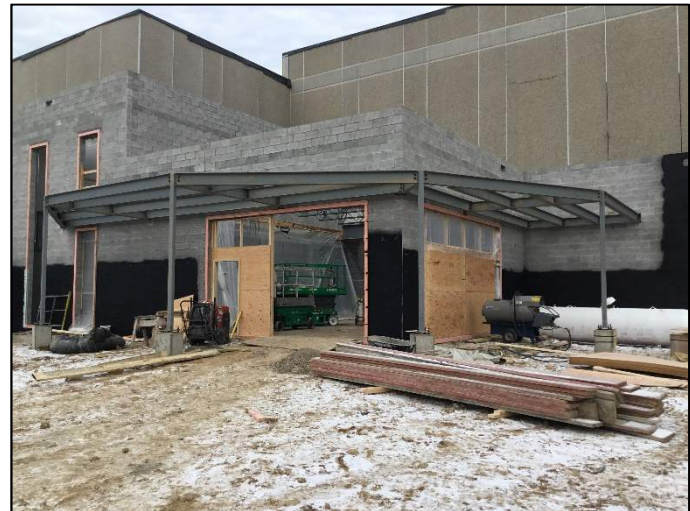
The vestibule overhang steel structure is complete. This overhang will be finished with metal coping around the edge, and slotted metal panels underneath.
